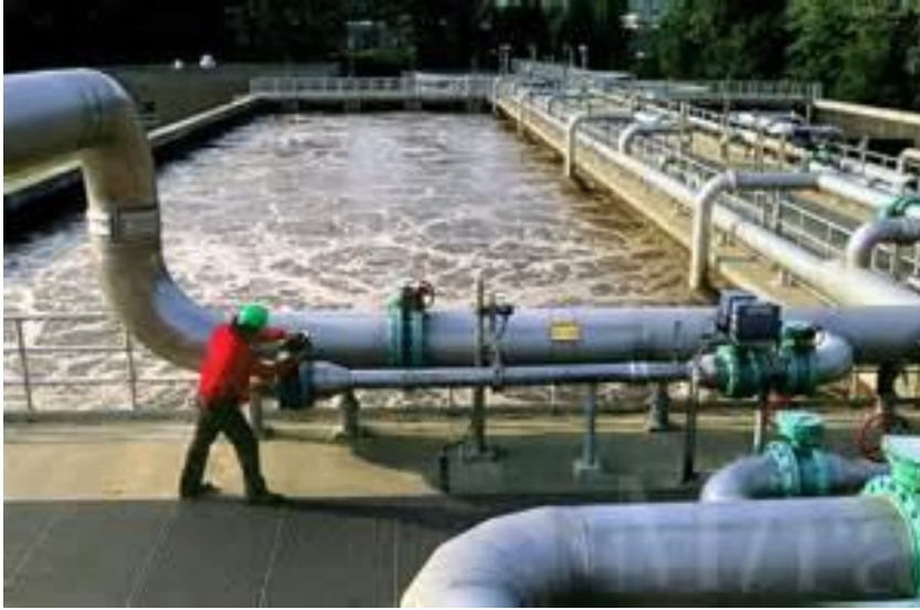
Figure 7. Municipal sewage treatment works using mussel shell to “polish” effluent.
